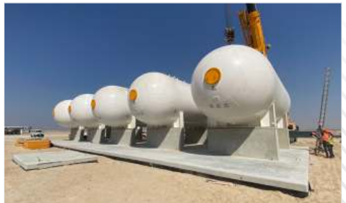
104 KL LPG Storage Vessels for Saudi Arabia
